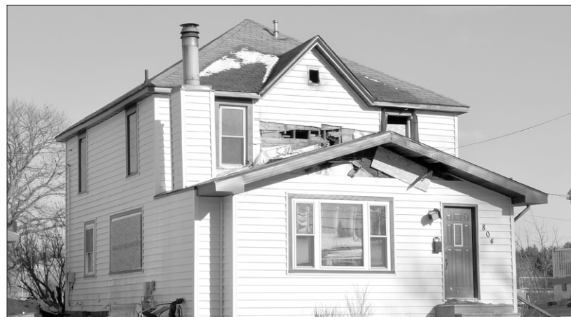
The Runge family's home at 804 Blackhawk Street in Reinbeck was destroyed by fire, and is a 'total loss' according to Reinbeck Fire Chief Jamie Eiffler.
